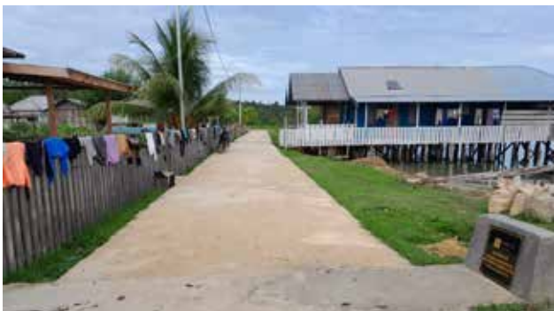
Pembuatan Jalan Rabat Beton Desa Kelo Construction of Kelo Village Concrete Rabat Road
