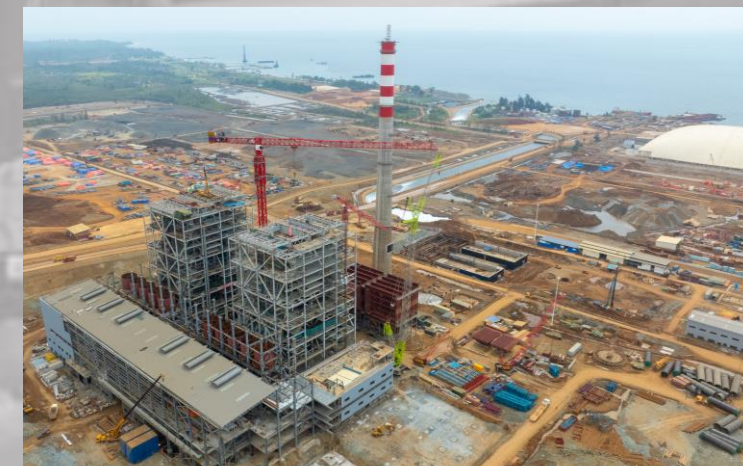
Power plant 3x380 MW to support KPS project (end of April, 2024 - 32.5% completed)
